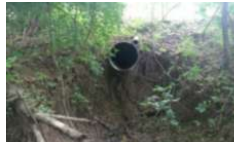
Figure B.1. The above outfalls are examples of different types of outfalls that must be identified on MS4 maps and included in the permittee’s screening program. Areas with highly developed land uses (e.g., commercial business complexes, aging infrastructure) have a greater potential to pollute and must be prioritized. Structural stability and erosion concerns should also be identified as part of an effective IDDE program.
